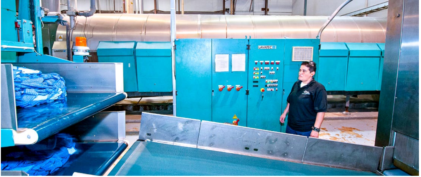
Division Laundry in San Antonio has added an assortment of LAVATEC equipment since buying their first continuous tunnel wash system in 1995 that is still in operation today.
