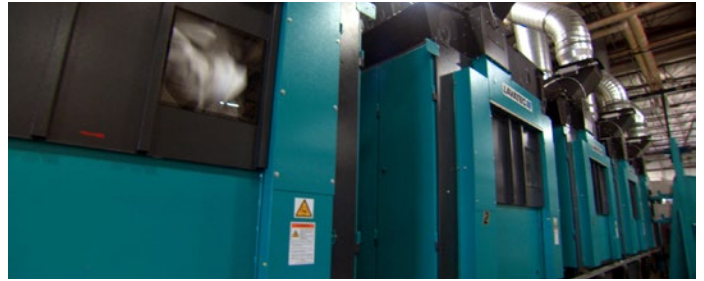
Five TT 745 natural gas dryers are part of Midwest Laundry's new Lavatec tunnel system. Early reports from Sodexo and UC Health say that dry times have been reduced by half (or more) for many linens – with significant energy savings.
