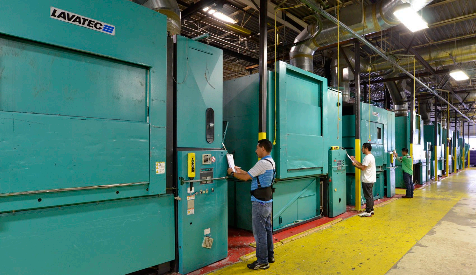
Twenty-three Lavatec 440-pound capacity dryers are employed in the three JVK facilities.
